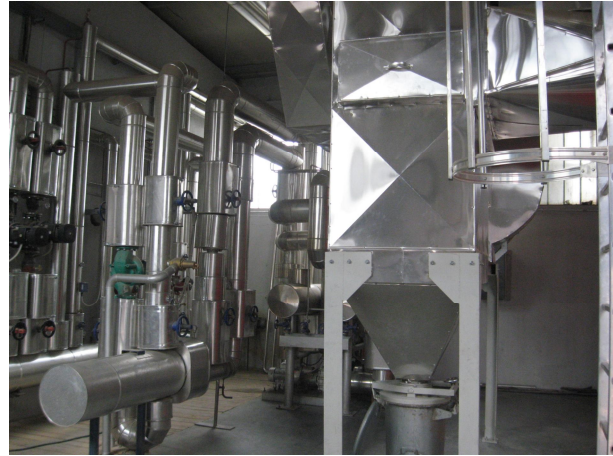
Picture 2: The heating system of Promming.
