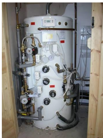
Domestic accumulator drawing heat from a wood burning stove and solar thermal array, with electric emersion coils for frost protection when owner is away in winter
