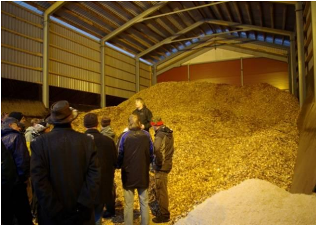
Figure 3: A chip store (boiler right behind the wall). Photo: Jyrki Raitila, VTT.
