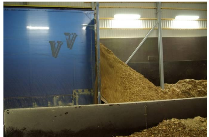
Figure 7: Chips being delivered; the truck has bar conveyors for unloading. Photo: Jyrki Raitila, VTT.
