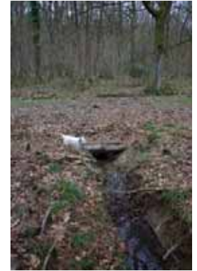
Figure 3: Simple culvert to prevent track lying wet during the winter and spring
