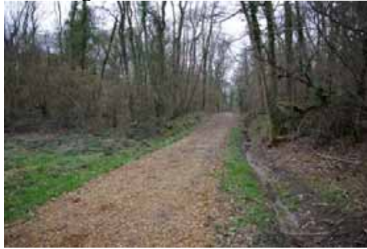
Figure 2: Access track improvement along a particularly wet section. Grants are only provided where there is a clear benefit in addressing a long term barrier to the woods sustainable management.
